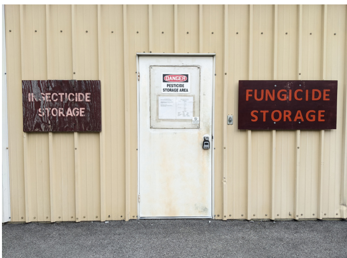
Figure 1. Clearly marked pesticide storage area.
